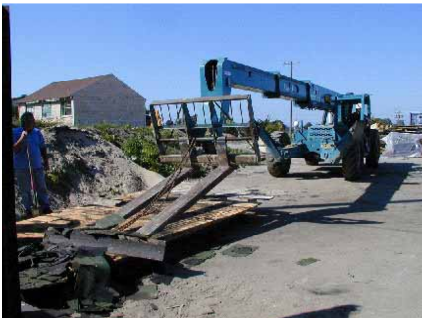
Figure 2.4 Using a “snowplow” to remove asphalt roof shingles. Finding fast, economical tools and methods for Deconstruction is a key step to making it standard practice.
