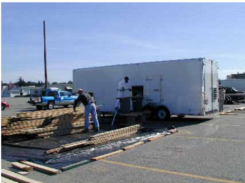
Figure 2.11 Trailer is parked at the deconstruction site, it is negatively pressurized to contain lead paint dust.
