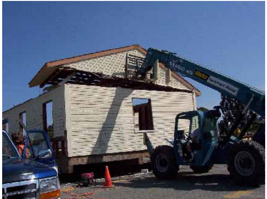
Figure 2.2 Roof is removed to ground level where it is safer and faster to deconstruct
